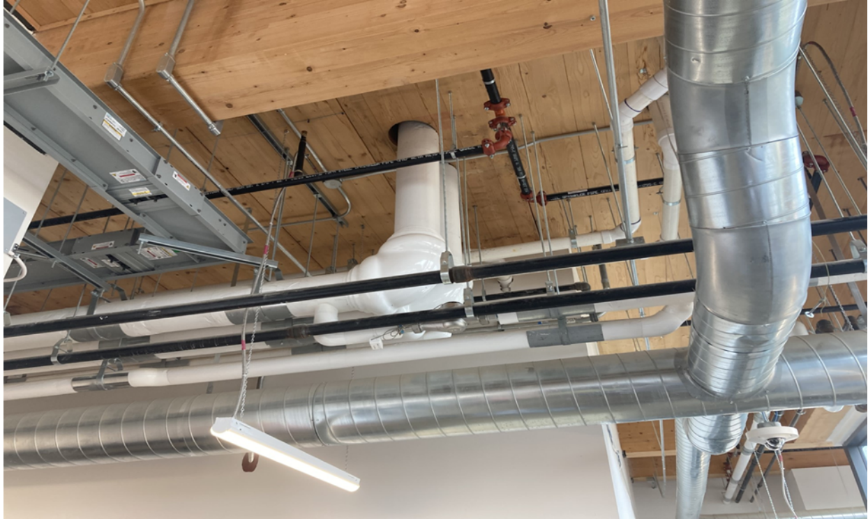
Figure 3. Overhead MEPFP Systems
